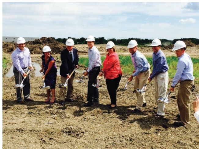
Photo 4-3. Breaking ground on a new building in Hobart's Northwind Crossing. Photo Credit: NWI RDA via Twitter.
